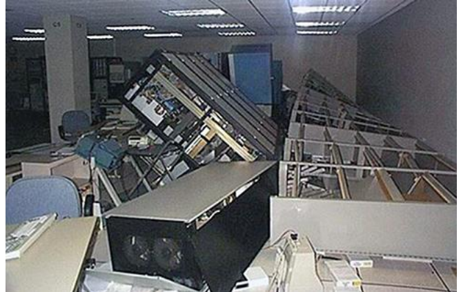
Abb. 2.21.2 &gt; Umgekippte Computerracks
